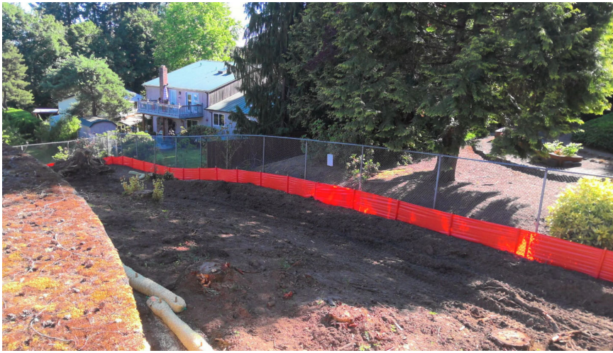
Erected temporary fencing for security and implemented erosion control to manage sediment runoff.
